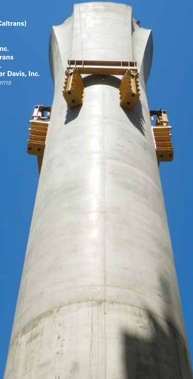
Figure 9 – Prefabricated pier brackets will support the falsework to construct the pier table. (Photo Courtesy of Tutor-Saliba)
