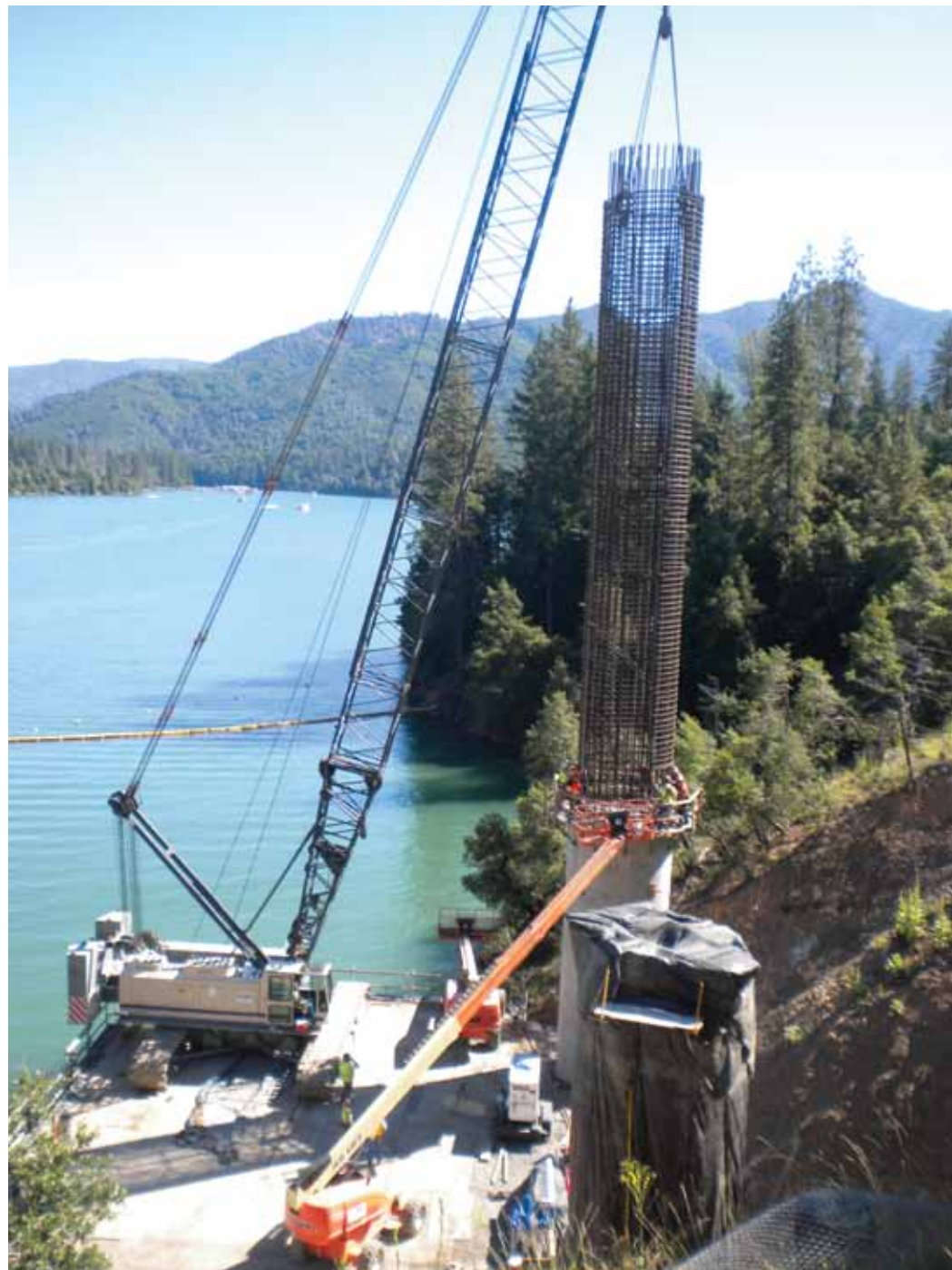
Figure 11 – Pier column reinforcing cage is being set in place as workers prepare to pour the first pier column. (Photo Courtesy of Tutor-Saliba)
