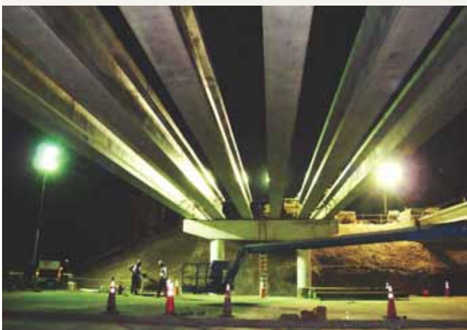
The replacement beams were designed within 12 hours, and the first beam was cast within 24 hours. Final beam designs were complete within 36 hours. Erection continued at night to ensure the deadline was met.
