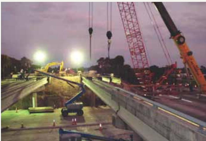
High-strength concrete with an 8500 psi design compressive strength was used to facilitate fabrication and delivery of the precast, prestressed concrete AASHTO I-beams, including 16 Type IV beams (12 at 99.5 ft long and four at 36.75 ft long) and four Type II beams (at 36.75 ft long).
