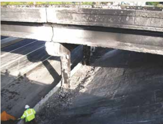
A fatal accident involving an 8200-gal. gasoline tanker badly damaged the Beachline Expressway/SR 528 overpass in Brevard County, Fla. The bridge was repaired with precast concrete girders in approximately 3 weeks. All photos: Lane Construction Corp.
