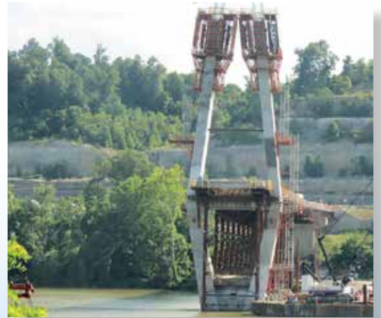
View from the Ohio Riverbank Facing Down Station. (Photo Courtesy of Brayman Construction Corporation)
