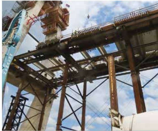
Deck Pans on the Kentucky Backspan. (Photo Courtesy of Brayman Construction Corporation)
