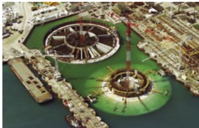
Below: The bases of the concrete pylons—the rafts—were constructed in dry docks. Two bases were constructed at a time.
