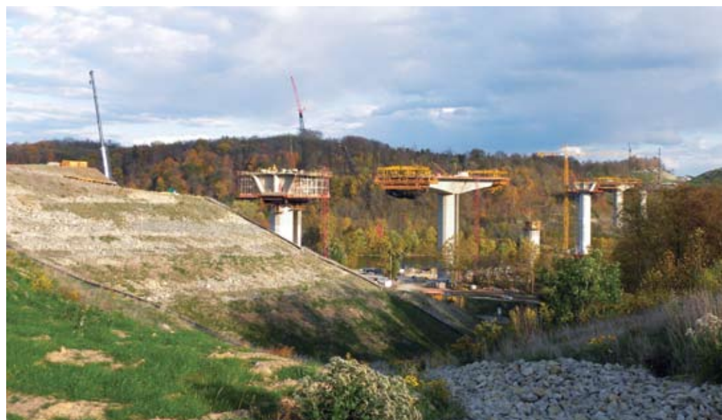
Figure 2 – October 2010 – Long cantilevers of the 51H Monongahela River Bridge are beginning to take shape as construction progresses on the Pennsylvania Turnpike Commission's newest segmental bridge. (Photo Courtesy of FIGG)
