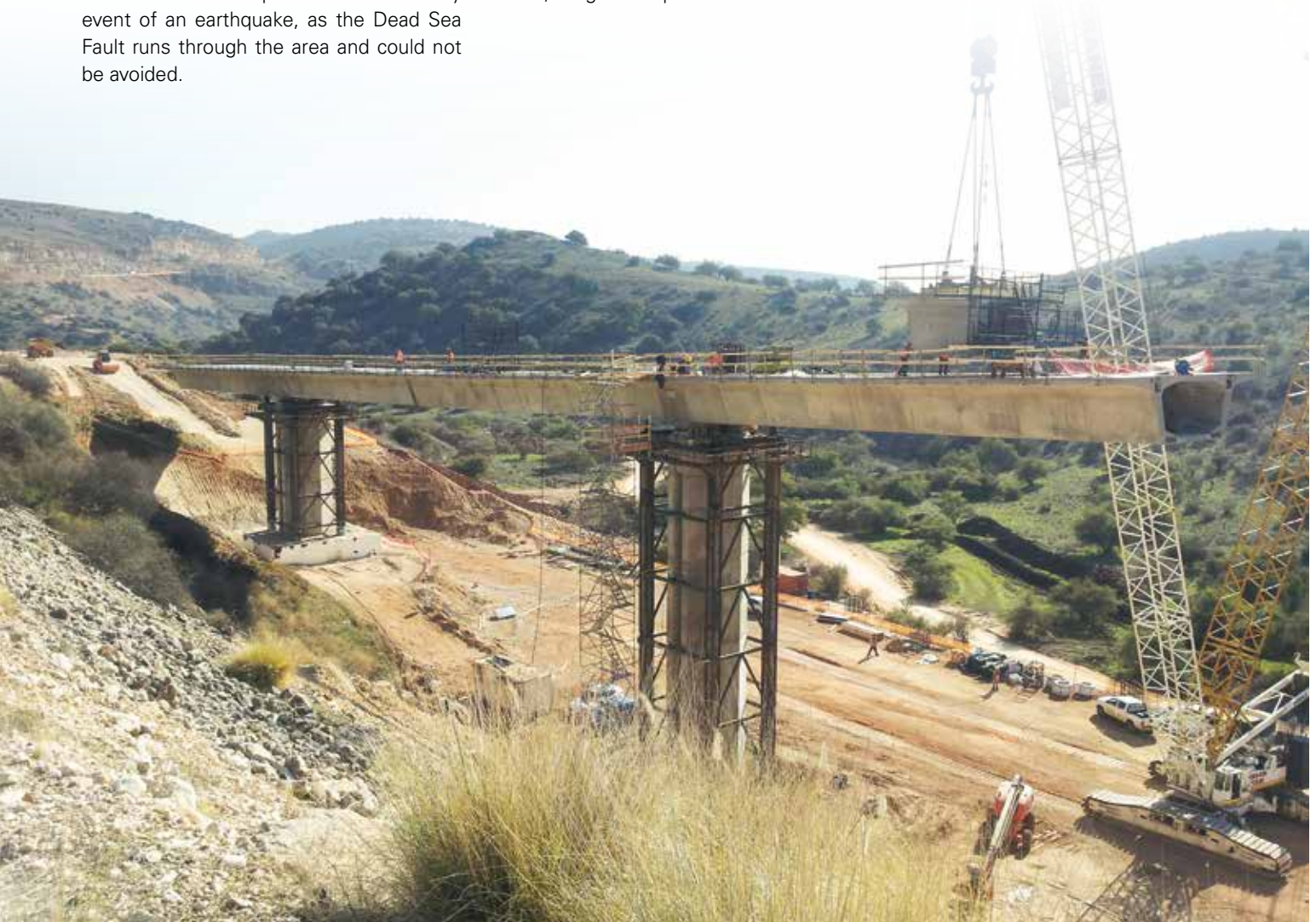
Amud bridge from the cantilever 5, last segment. (Photo Courtesy of Shikun & Binui - Solel Boneh Building & Infrastructure Ltd.)
