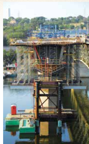
Figure 11 – US 281 Colorado River Bridge over Lake Marble Falls. (Photo Courtesy of Archer Western Contractors)
