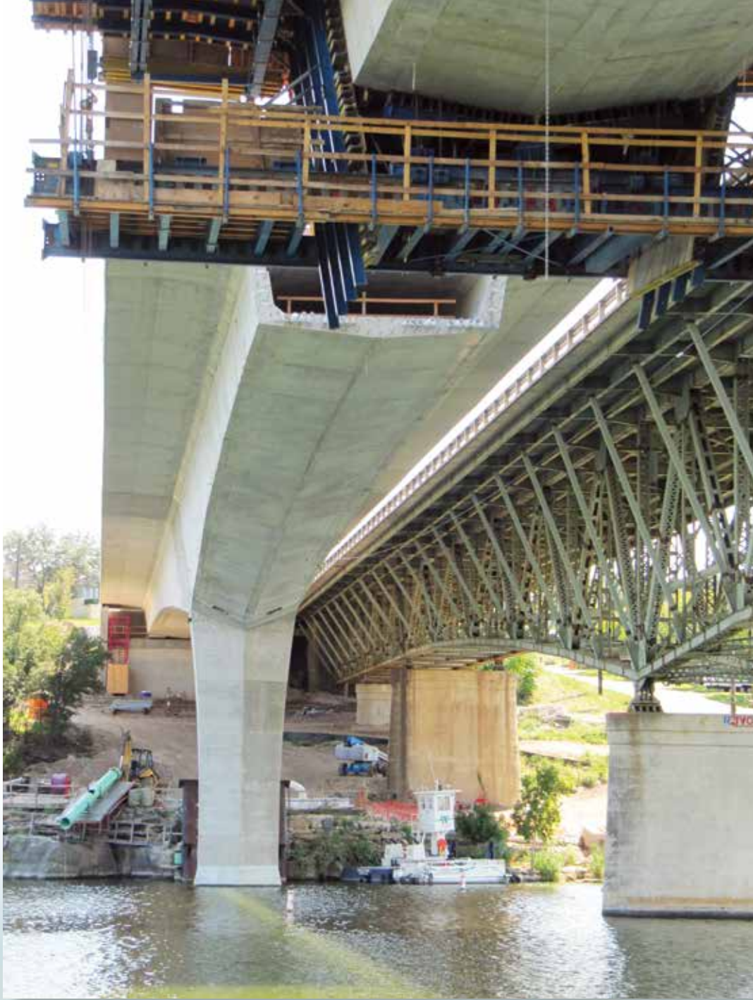
Figs. 12 and 13 – US 281 Colorado River Bridge over Lake Marble Falls. (Photo Courtesy of Archer Western Contractors)
