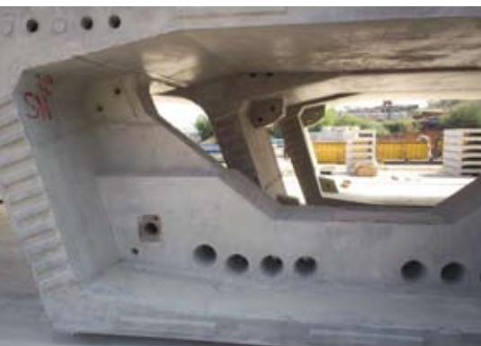
Deviation segment featuring post-tensioning tendon diabolos in the foreground. Photo: Finley Engineering Group Inc.
